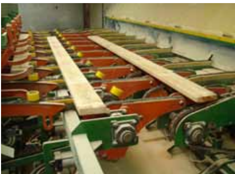
Above: A dual-actuating smart drop out gate directly behind the trimmer drops out selected boards for rerouting.
