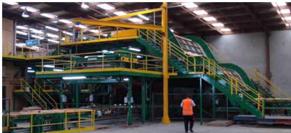
A new USNR double radius-back unscrambler is situated just upstream of the grading area.
