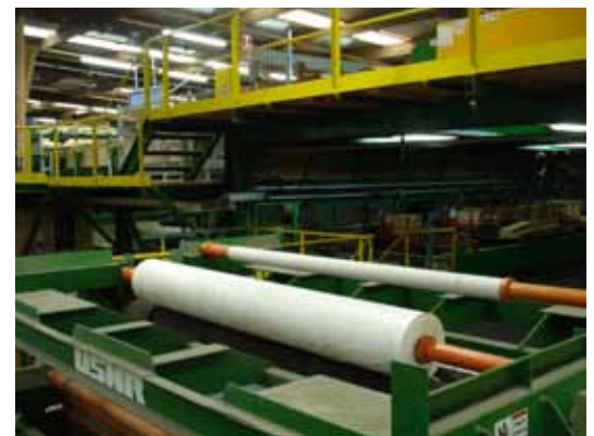
A new triple paper feeder and cutter was also installed.
